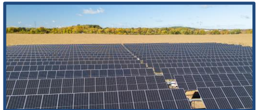
Badger Hollow Solar Farm (300 MW) located near Cobb and Montfort
